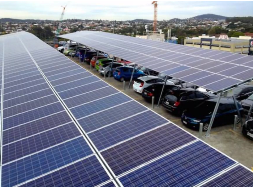
PHOTOVOLTAIC SOLAR CAR PARK SUNSHADING AWNING
